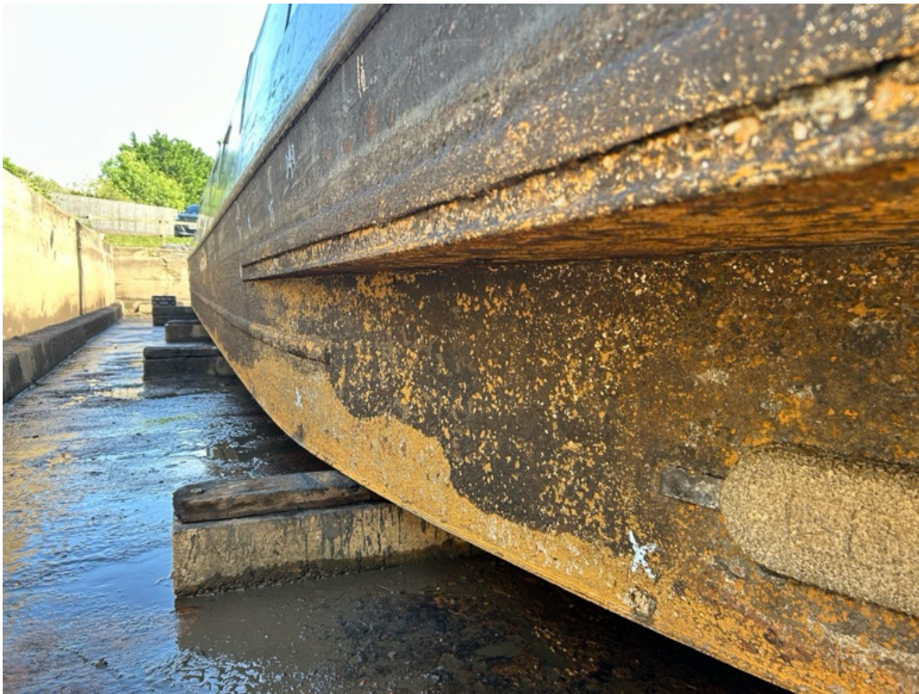
This 20-year old narrowboat has had no maintenance and was covered in pitting. The base plating was covered in over an inch of thick growth / debris / corrosion scaling
