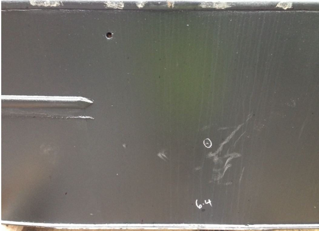
This 1992 narrowboat was grit-blasted and epoxy coated from new. In 2014 it was surveyed and found to have only x 1 pit at 1.5mm.
